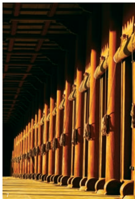
7. A series of 20 entasis columns adorn the front facade of the Main Hall of Jongmyo.
